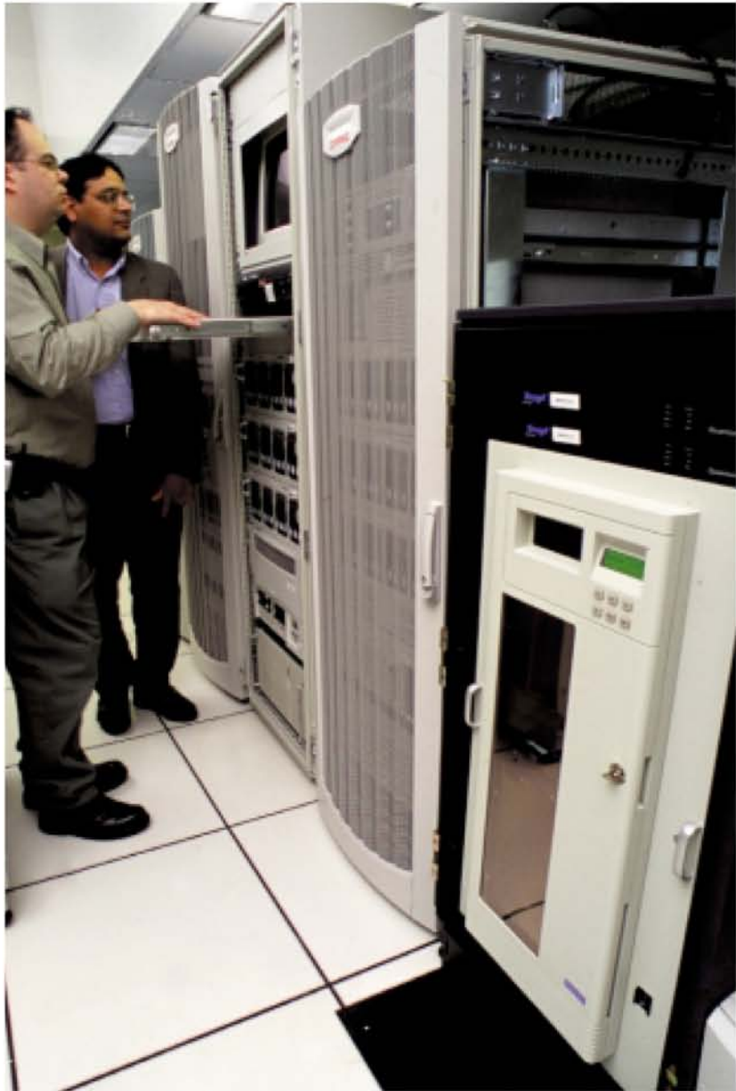
Sonty and Feldman at work in ANALYTIC i 's data center. The company currently handles a total data load of four terabytes, and depends on Qualstar's TLS-8222 library, running LTO tape drives, to seamlessly handle backups and restores with ease, speed and reliability.
